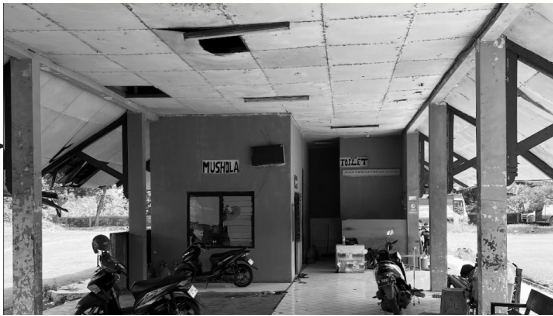
Insufficient Facility Condition
