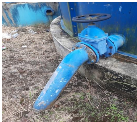
Gambar 4. 15 Pipa Distribusi Pelanggan
