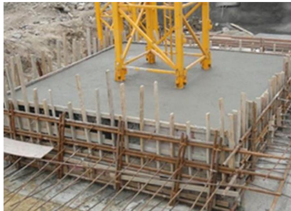
Gambar 3.5 Base Tower Crane
