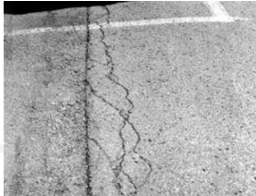
Gambar 3.11 Tingkat Medium Kerusakan Edge Cracking (Sumber: Department of the Army, 1982 )
