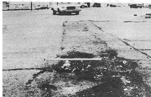
Gambar 3.21 Tingkat High Kerusakan Patching and Utility Cut Patching
