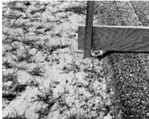
Gambar 3.13 Tingkat Low Kerusakan Lane/Shoulder Drop-Off (Sumber: Department of the Army, 1982 )
