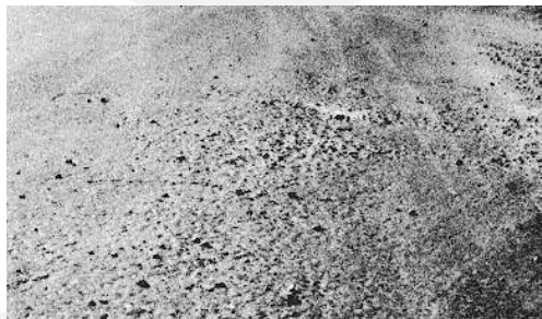
Gambar 3.30 Tingkat Medium Kerusakan Weathering and Raveling
