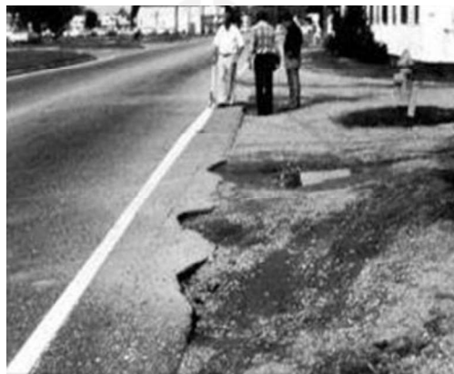
Gambar 3.12 Tingkat High Kerusakan Edge Cracking (Sumber: Department of the Army, 1982 )
