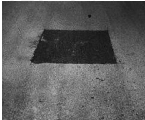
Gambar 3.19 Tingkat Low Kerusakan Patching and Utility Cut Patching
