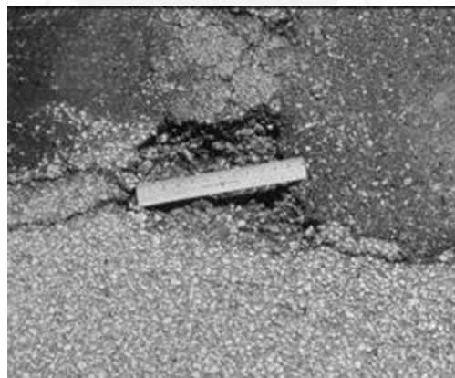
Gambar 3.23 Tingkat Low Kerusakan Potholes (Sumber: Department of the Army , 1982)
