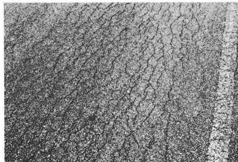
Gambar 3.2 Tingkat Medium Kerusakan Alligator cracking (Sumber : Department of the Army, 1982 )
