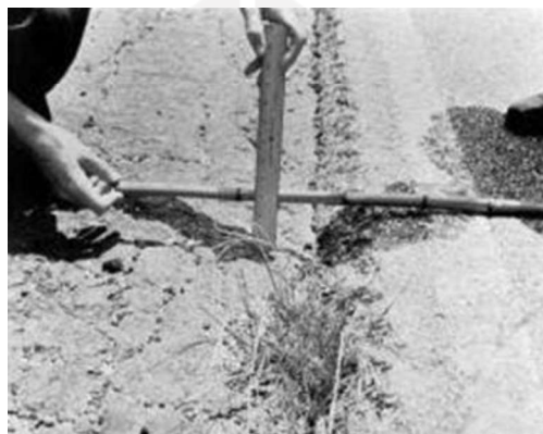
Gambar 3.14 Tingkat Medium Kerusakan Lane/Shoulder Drop-Off (Sumber: Department of the Army, 1982 )
