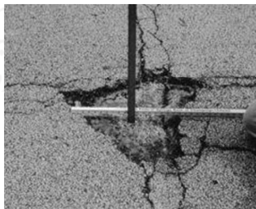
Gambar 3.24 Tingkat Medium Kerusakan Potholes (Sumber: Department of the Army , 1982)
