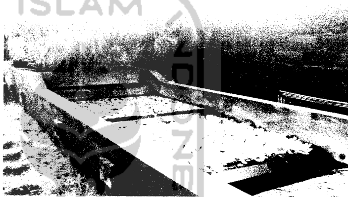
Gambar 2.3. Bangunan horizontal sand filter plant
