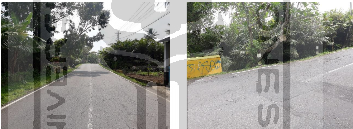
Gambar 1.2 Cracking Perkerasan Jalan (Tempel-Pakem)
