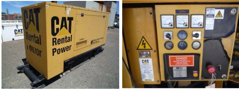
Gambar 5–19 Silent Generator Caterpillar 100kVa
