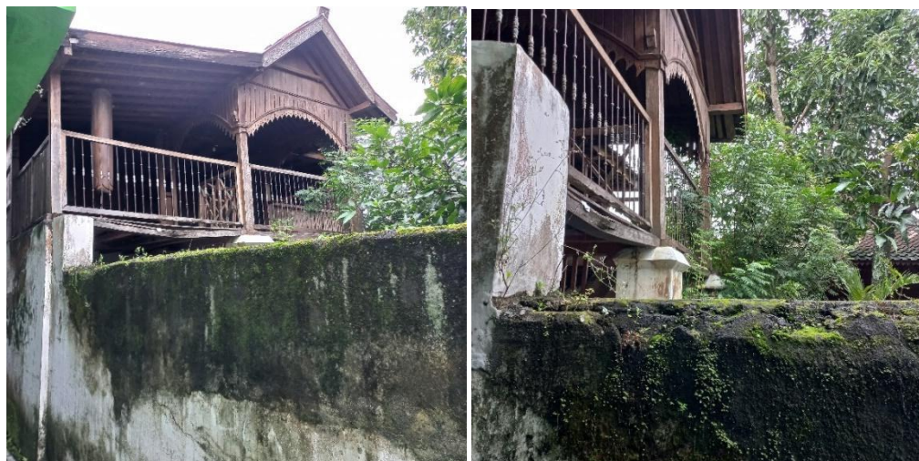
Figure 2 Cutted Wall (Pictures taken by author)
