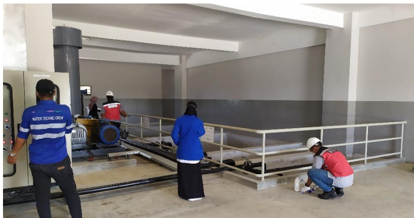
Gambar 4.2 Sewage Treatment Plant (STP) Bandara Internasional Yogyakarta
