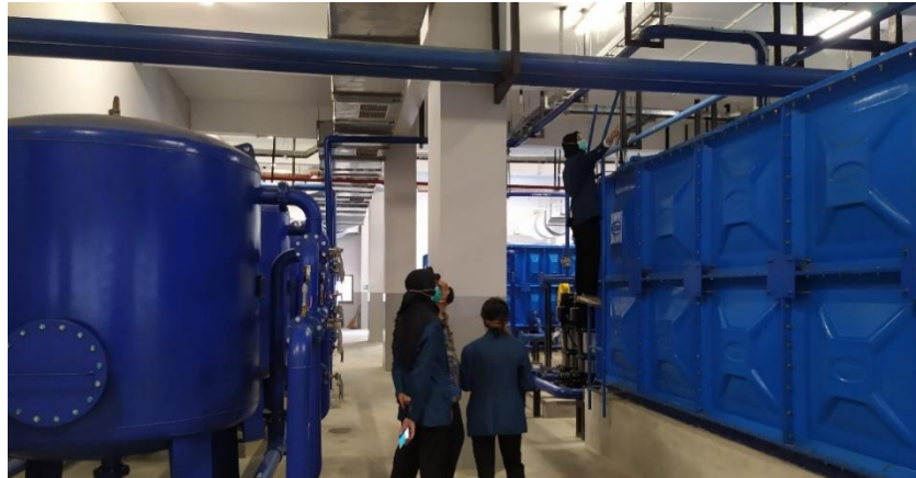
Gambar 4.1 Ground Water Tank (GWT) Bandara Internasional Yogyakarta
