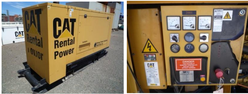
Gambar 5–19 Silent Generator Caterpillar 100kVa
